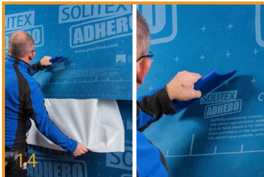
14 Overlap the Membrane Layers Apply all the remaining membranes - one by one - horizontally in an overlapping, waterproof manner. The minimum overlap for membranes is 150 mm.
