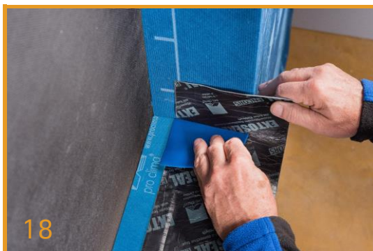
18 Apply Sub Sill Flashing - TESCON EXTONSEAL® TESCON EXTONSEAL® Sill Tape should extend minimum 100 mm up the jambs. The corners of the TESCON EXTONSEAL® are stretched & adhered into place.
