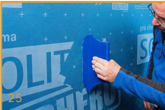
Repair Using SOLITEX EXTASANA ADHERO® As an alternative, defects can also be repaired by adhering a piece of ADHERO onto them. Smooth adhesive joints firmly using a PRESSIFIX.
