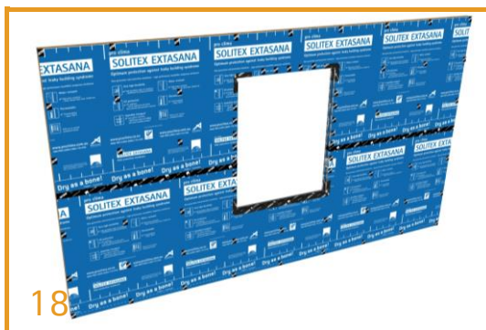
Basic Install Completed Around Openings SOLITEX EXTASANA®, TESCON EXTORA® and TESCON EXTOSEAL® form a continuous system. Any damage or tears should be patched with TESCON EXTORA®.
