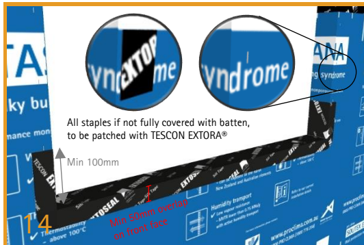
Applying TESCON EXTOSEAL® Sill Tape TESCON EXTOSEAL® Sill Tape should extend minimum 100 mm up the jambs. The corners of the TESCON EXTOSEAL® are stretched & adhered into place.
