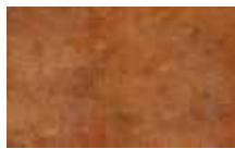
FCR 504 535 Thick rust
