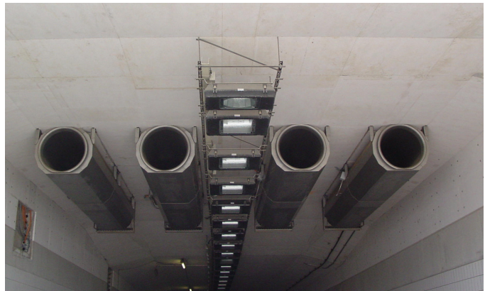
Figure 13: anchor system for jet fans
